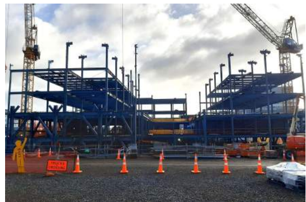
Major progress: a view of Tōtara Haumaru from the entry side of the building.
